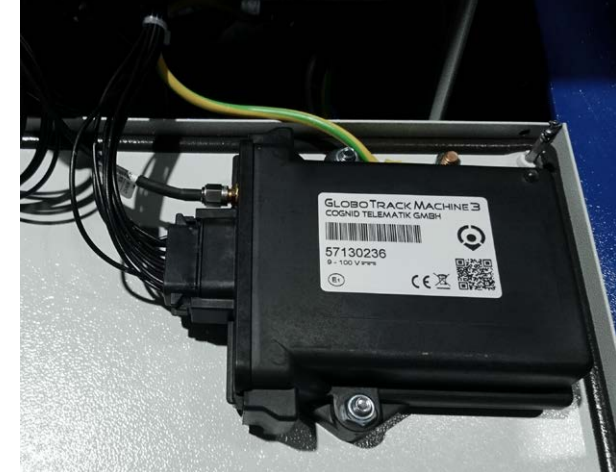
GTM installation on the cover of the switch box and connection to the Avermann circuit board
