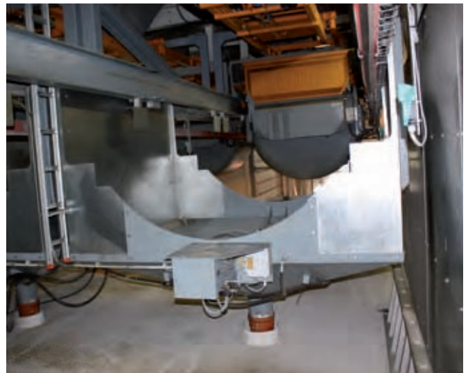
Cleaning station for the bucket tracks
