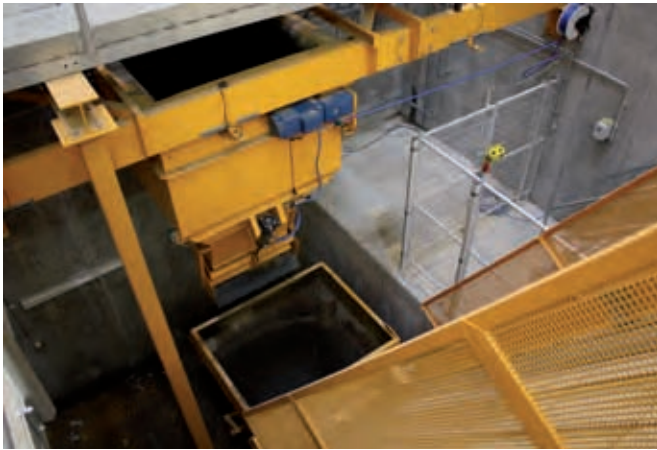
Transfer of the aggregates to the three inclined bucket elevators
