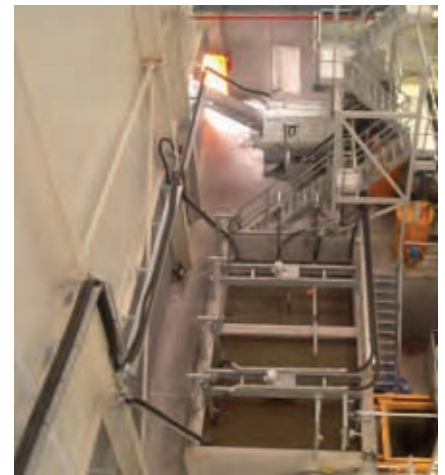
Overview of the Bibko plant equipment in the BLANDE ANLÆG area. Agitation tank 1 can be seen above, agitation tank 2 below
