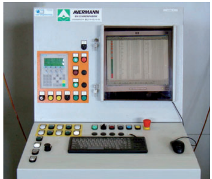
Control panel – storage and retrieval unit
