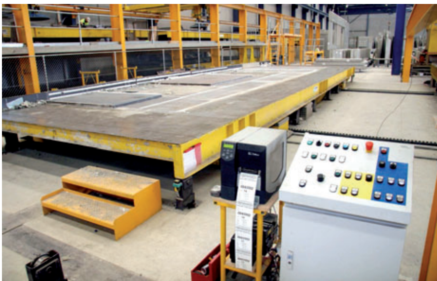
Tilting bay control panel and label printer
