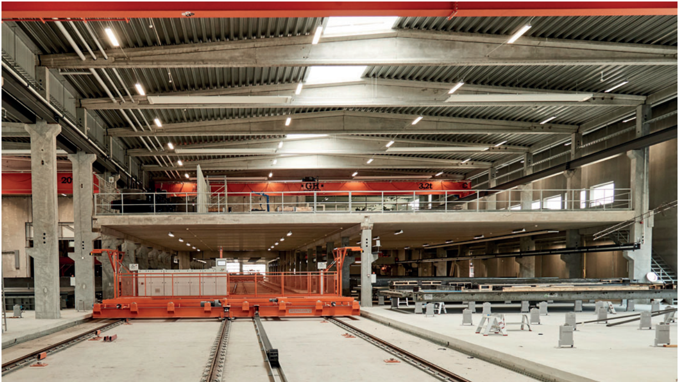
Fig. 3: Pallet transport using a central transfer platform
